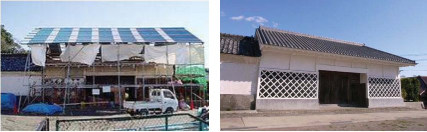
Fig. 1 - Nagayamon under repair work (left), and after repairmen (right) (photograph by Okusu Ecomuseum).
